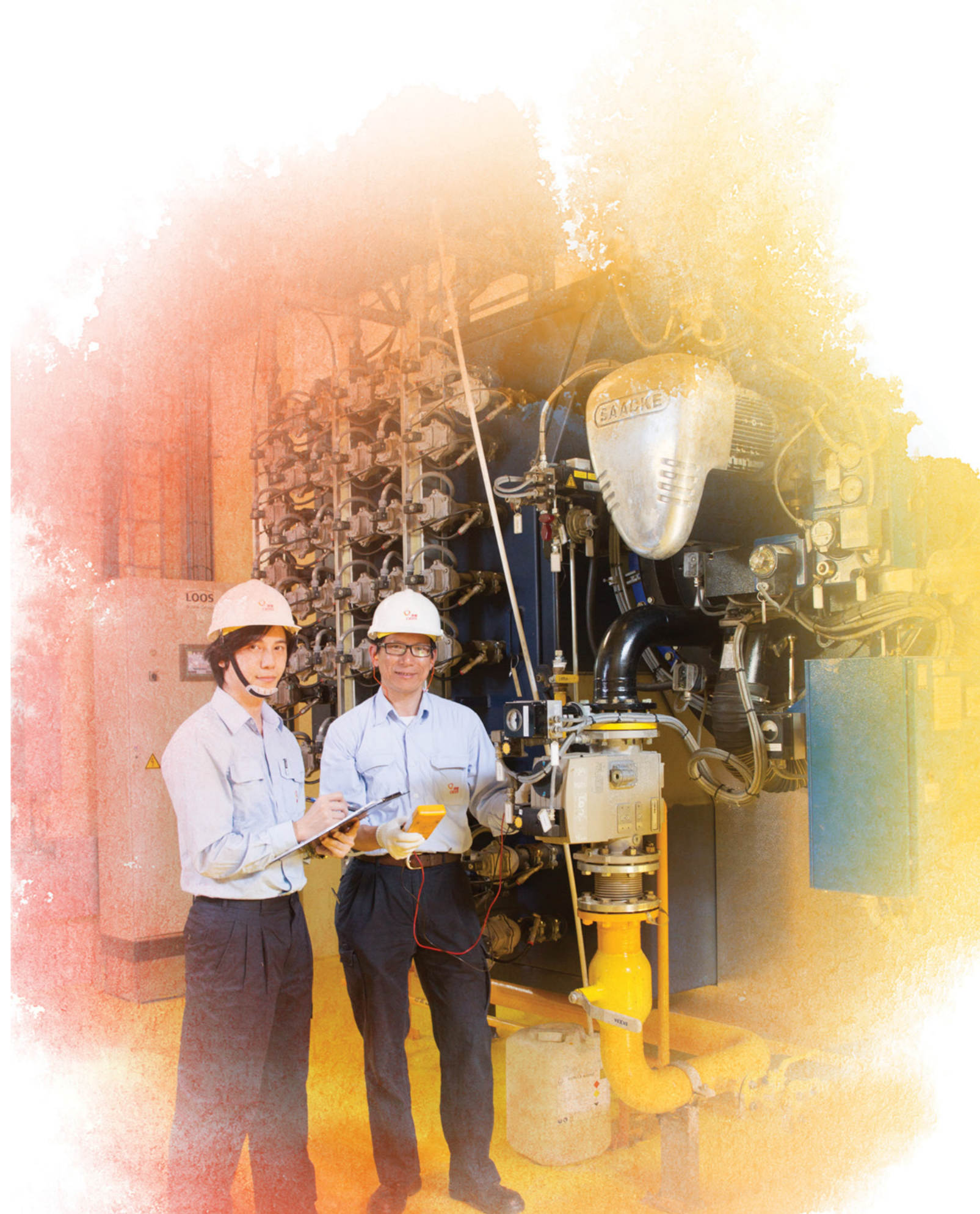
工程師林耀輝 (左) 及高級技術操作員陳華根 (右) 於輔助鍋爐 O Engenheiro Lam Io Fai e o Operador Técnico Sénior Chan Wah Kan junto à caldeira auxiliar Engineer Lam Io Fai and Senior Technical Operator Chan Wah Kan at the auxiliary boiler
